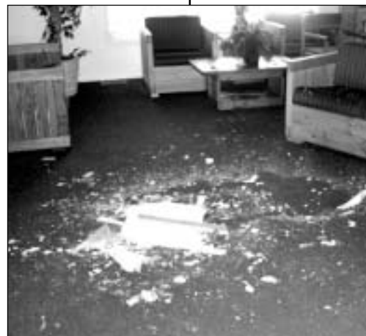
Water soaked through the ceilings and damaged everything below.
